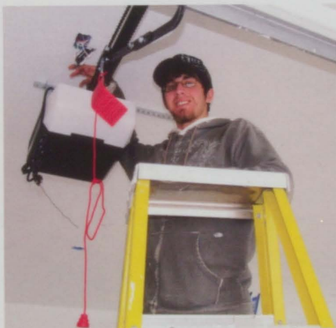
Senior David Markgraf works on installing a garage door opening sensor at Auburn during his construction class.
